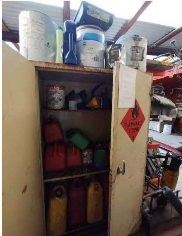
Photo 11: Flammable liquid depot in covered maintenance area in south west of the site
